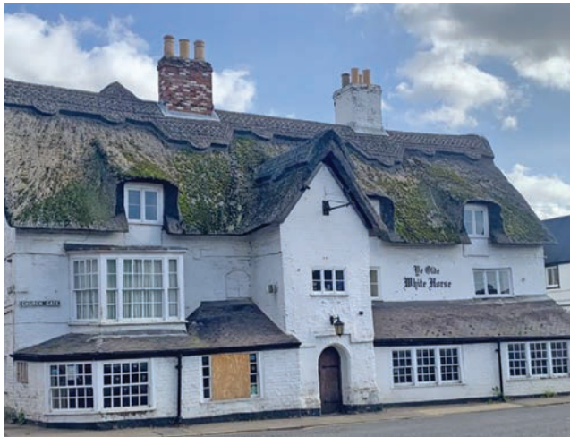
The White Horse public house is the only building that has retained a thatched roof
