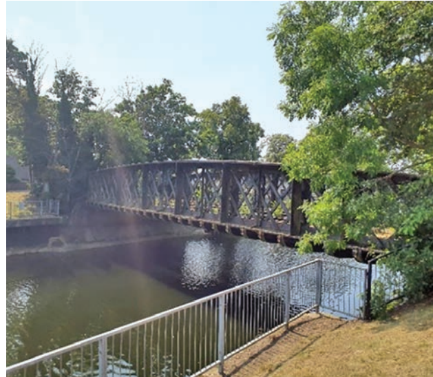
Disused Spalding to March railway bridge at the southern extent of the conservation area
